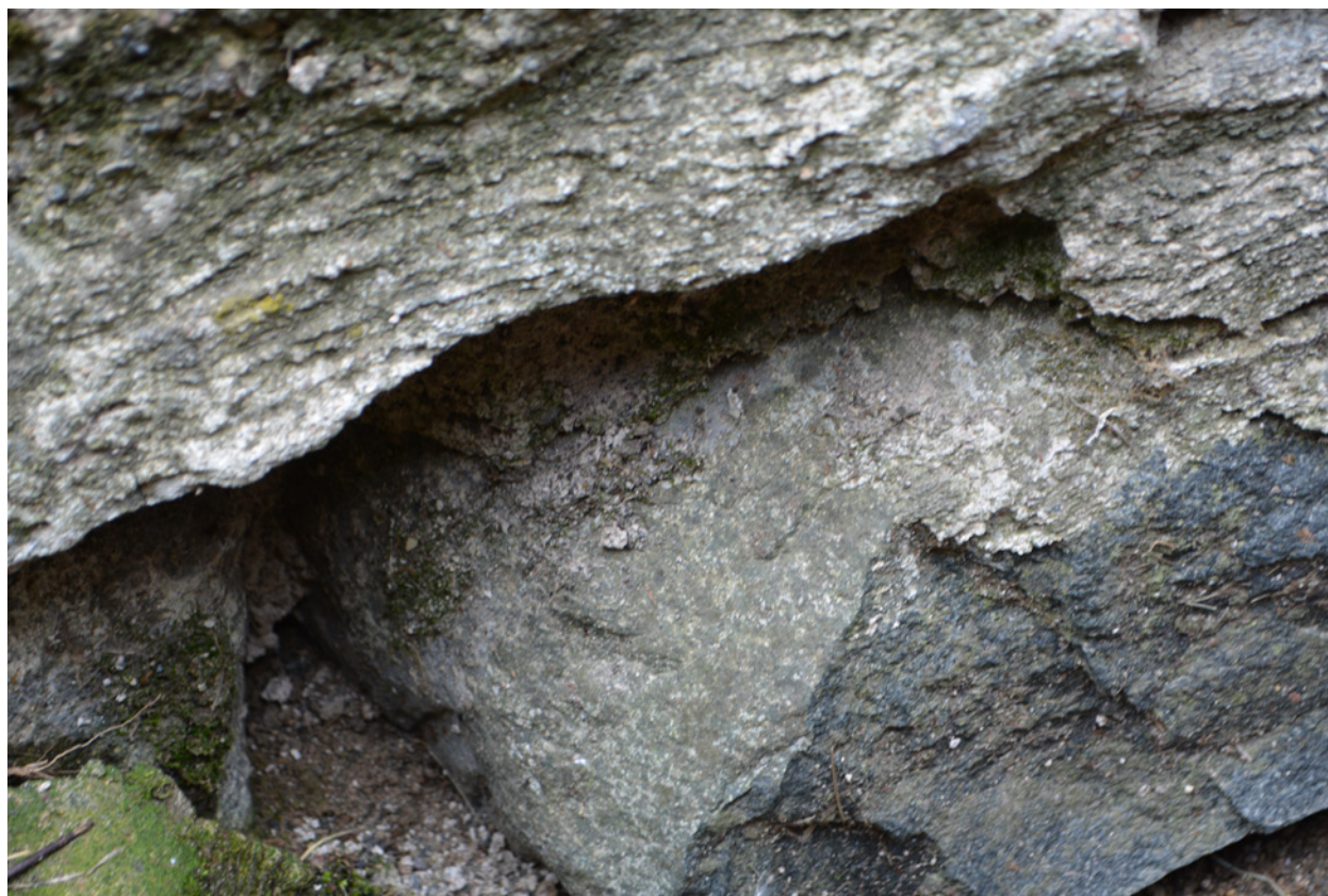
22 Example of deteriorated mortar at foundation wall, north elevation. June 2018.
