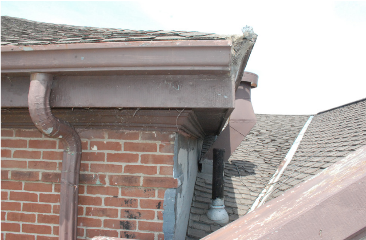
11 Improperly installed roof edge, southeast corner of the roof. June 2018.
