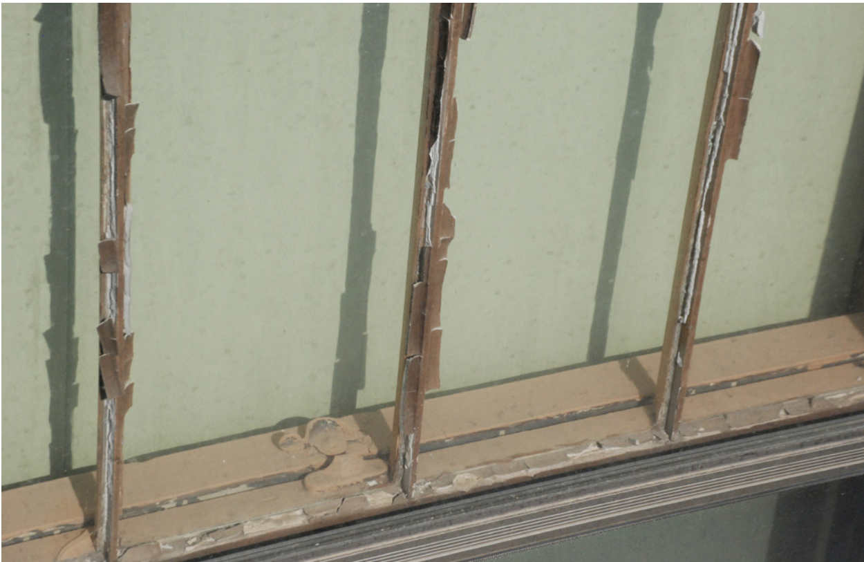
31 Typical deteriorated glazing putty at windows. June 2018.
