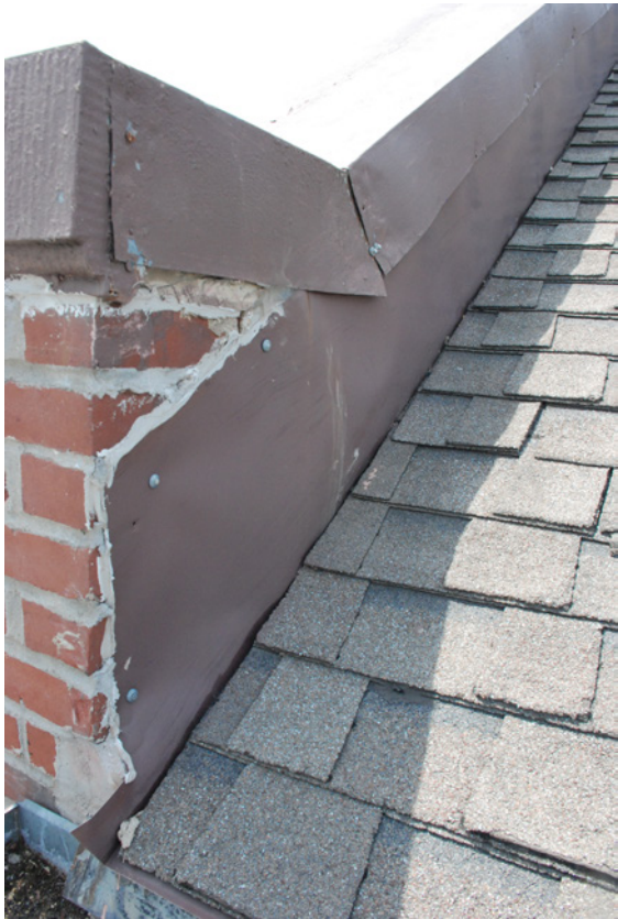
12 Improperly installed flashing at parapet wall. June 2018.
