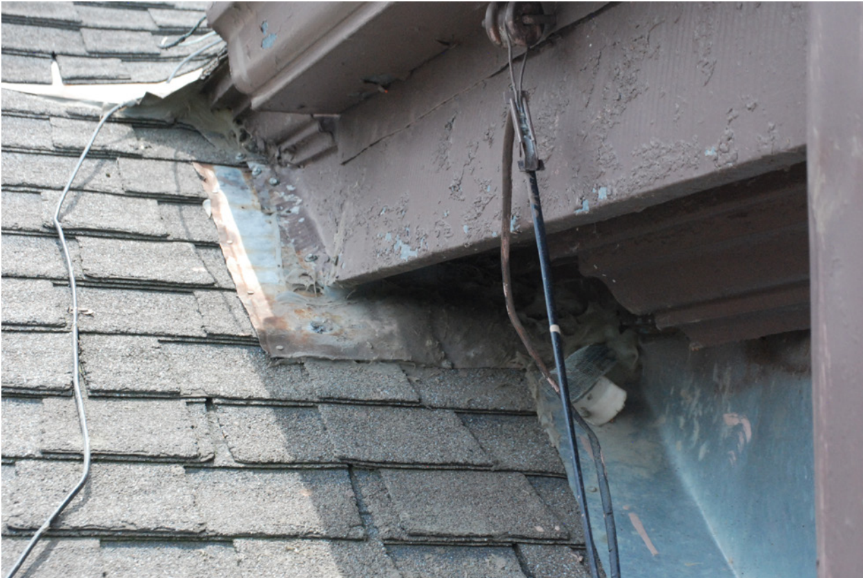
10 Example of improperly installed flashing. June 2018.
