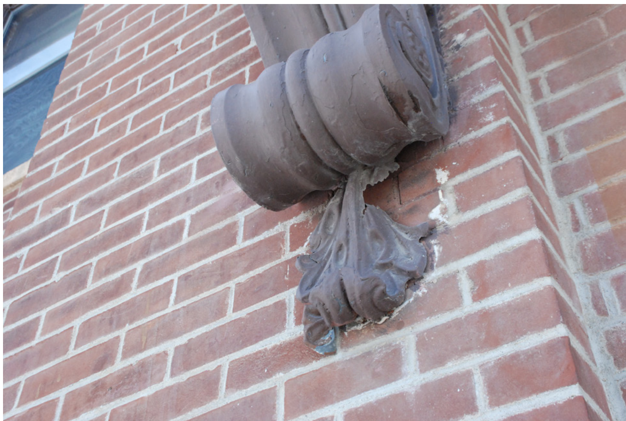
20 Area of missing metal at decorative acanthus leaf at main entry, west elevation. June 2018.
