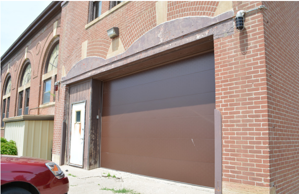
23 Existing doors and deteriorated concrete driveway at Firehouse, south elevation. June 2018.
