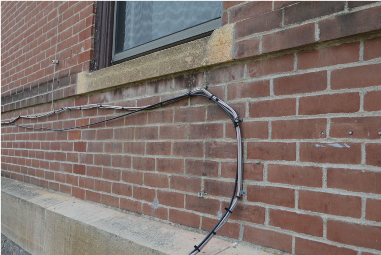
34 Typical wires attached to brick at north elevation. June 2018.
