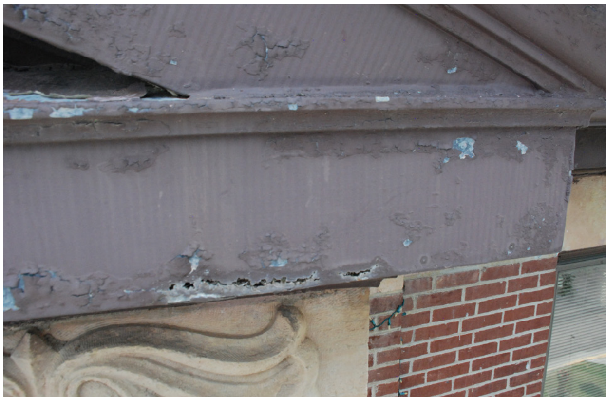
19 Area of deteriorated metal at pediment, main entry at west elevation. June 2018.
