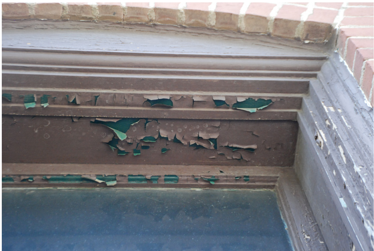
30 Typical deteriorated paint condition at windows. June 2018.
