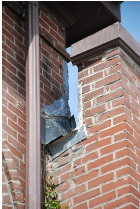
14 Intersection of wall between City Hall and Firehouse, missing flashing and conductor head. June 2018.
