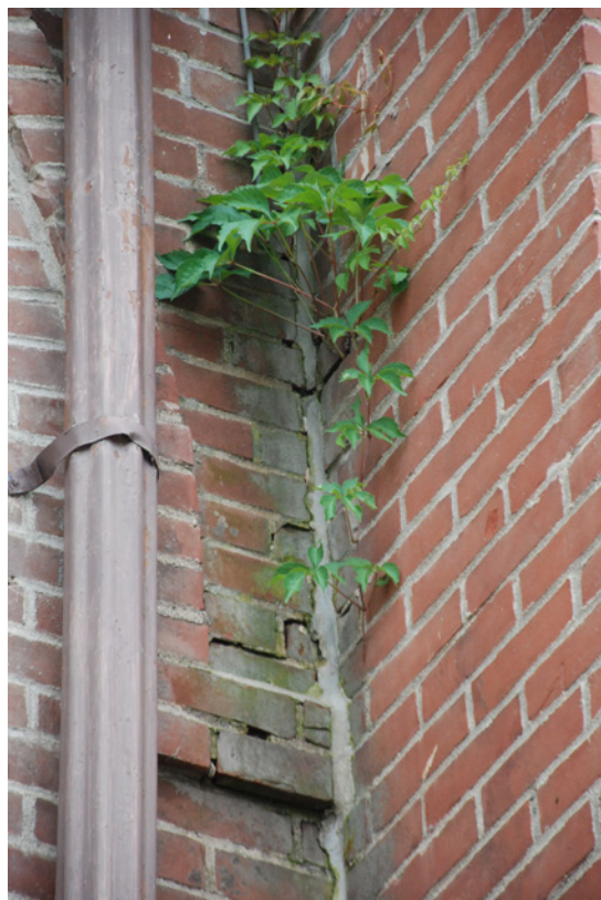
21 Deteriorated mortar joints at intersection between City Hall and Firehouse, south elevation. June 2018.
