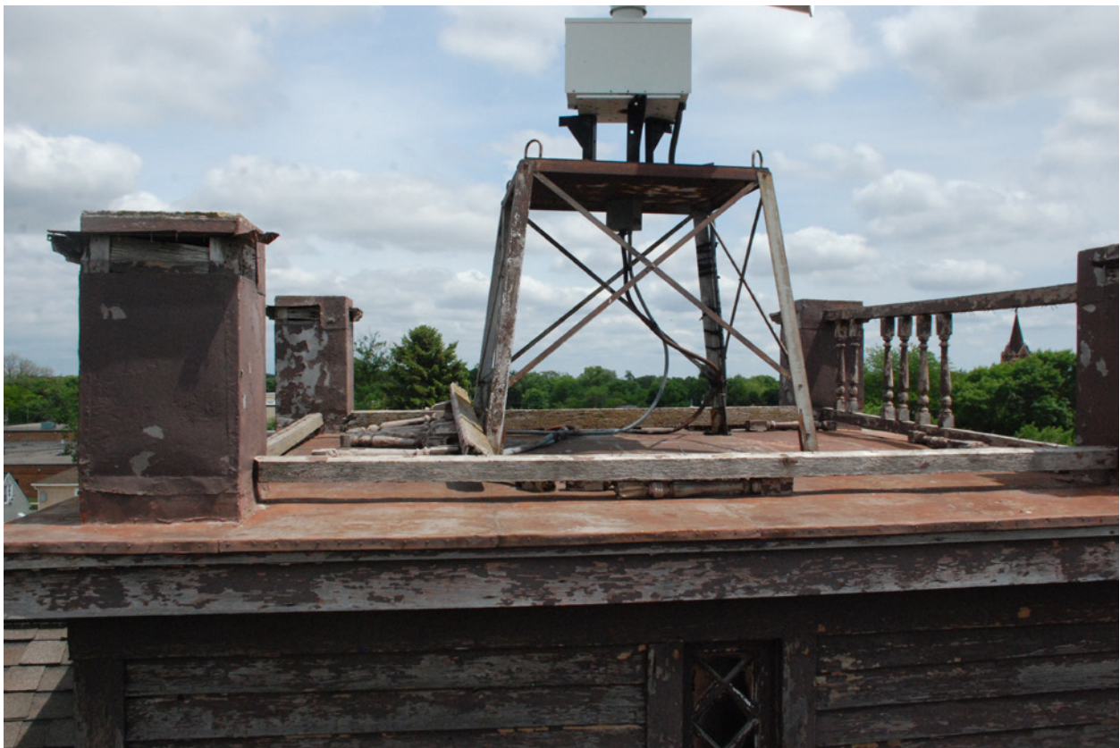
16 View of top of the tower. Note remaining balustrade and the existing weather siren. June 2018.
