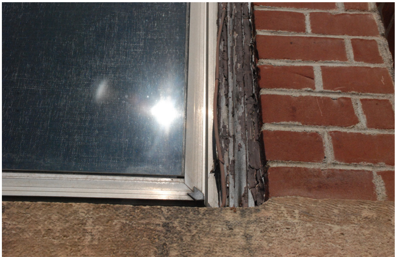
29 Typical condition of double-hung windows; metal storm window, deteriorated paint and wood casing. June 2018.
